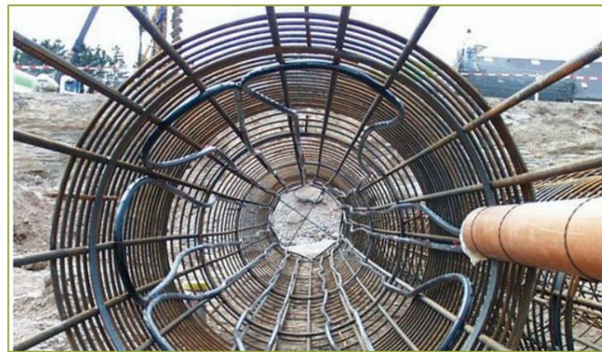
Pipes integrated into basements pillards
